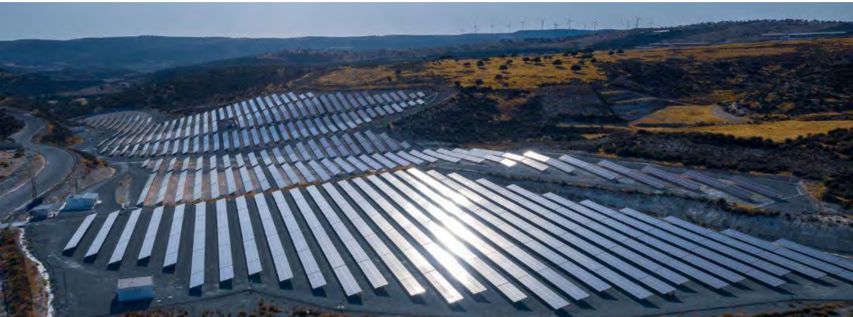
Photovoltaic installations in the town of Guillena, Seville.
