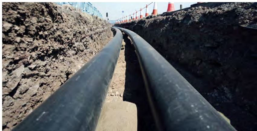
Community heating network in Midlothian, Scotland.
